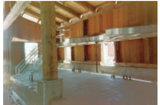
Nickel & Nickel Tank Pad with LeDuc & Dexter's soon to be hidden processed piping
