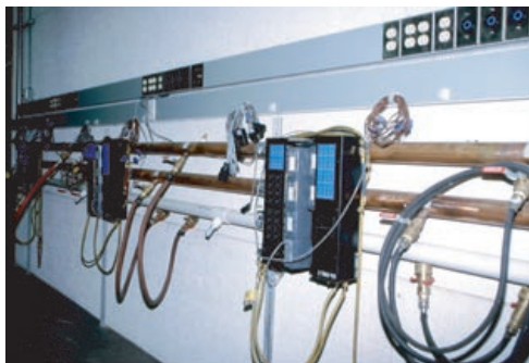
Cooling Water & Vent Piping at IGC Polycold Product Testing Stations
