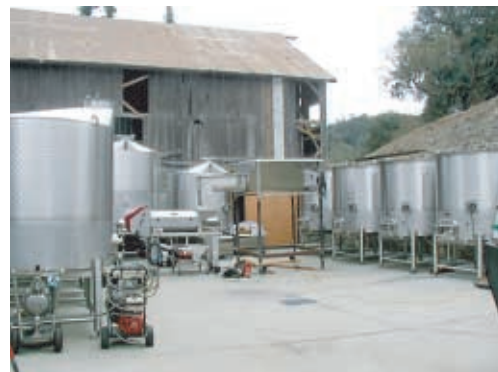
Cary & Associates Builders, Inc. assembled the Brown Estate Winery crush pad in time to crush 20 tons of Cabernet at the end of September 2002. The historic Brown Estate building is in the background.
